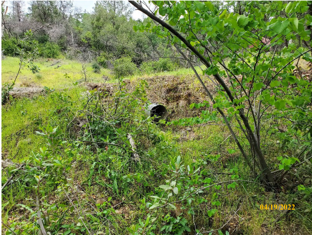
Photo 5. Site 122 : View looking upstream at the current CMP outlet and outboard fillslope for Site #'s 123 and 122. A new 24-inch CMP will be placed at the base of fill and will be adequately sized to transmit flow from both streams.
