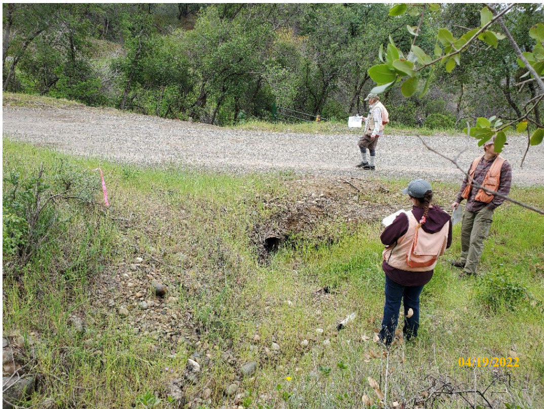
Photo 6. Site 122 : View looking downstream towards existing CMP inlet. Streamflow from Site #123 comes in from the right ditch and uses this CMP. The existing CMP is undersized to convey the streamflow from both streams.
