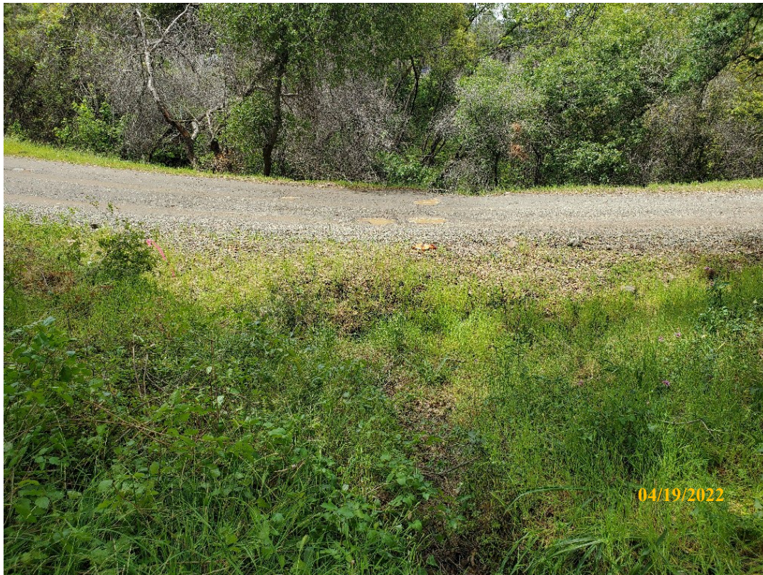
Photo 32. Site 139: View of current channel alignment and stream crossing surface. The CMP inlet is in front and to the left of the placed tape measure. The CMP is undersized and placed shallow in the roadbed causing infilling at the inlet and erosion at outlet.
