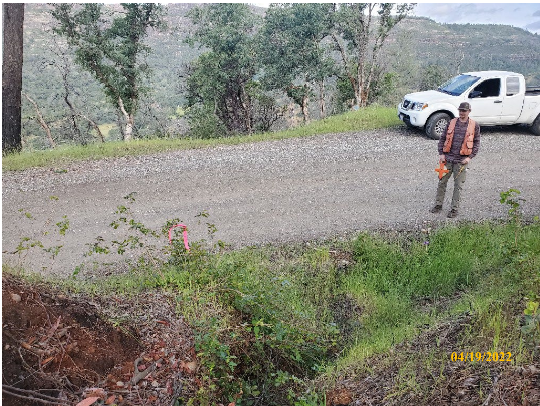
Photo 16. Site 129: View of the current CMP inlet and stream crossing surface. Long ditch and stream flow is conveyed through this undersized CMP causing erosion of the outboard fillslope at the outlet.
