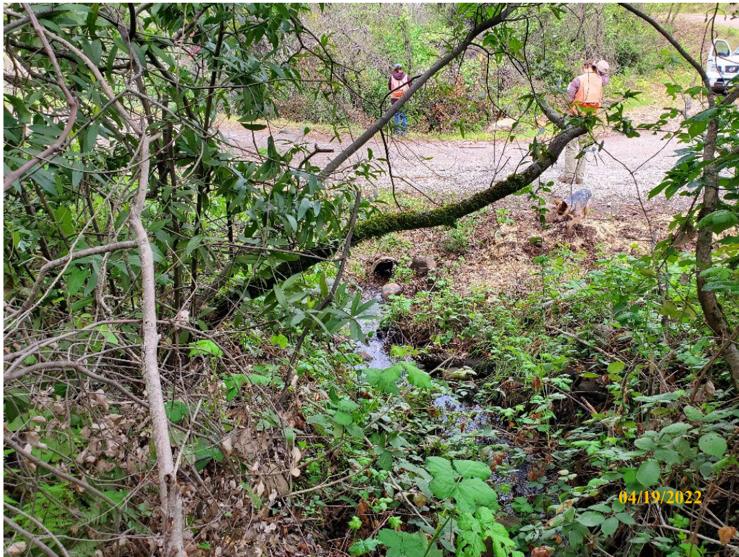
Photo 36. Site 142: View looking downstream at the current CMP inlet. The CMP is placed shallow in the fill and is relatively flat, increasing its potential to fill with sediment and plug.
