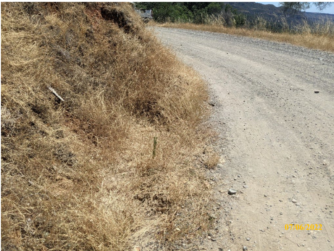
Photo 12. Site 127: View of inlet area of existing DRC#20. Standing in inboard ditch 12 feet uproad of inlet.
