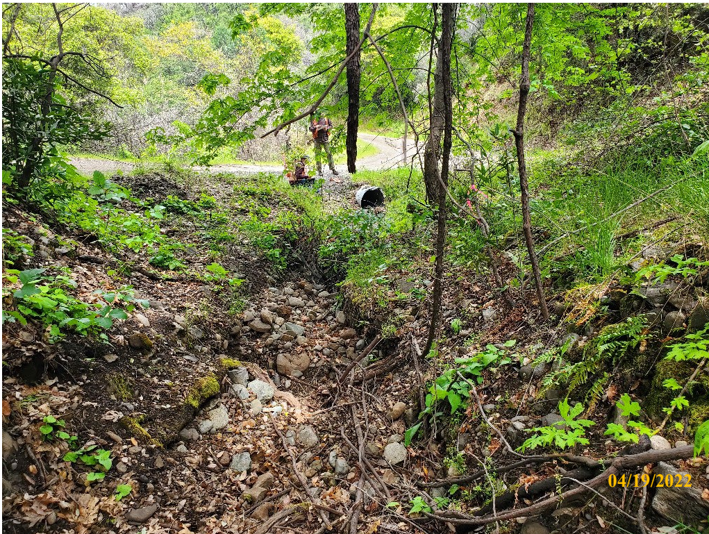
Photo 30. Site 138: View looking downstream at the current CMP inlet and channel alignment. The CMP is not in alignment with the stream channel and is also placed shallow in the fill exposing it on the outboard edge of the road.
