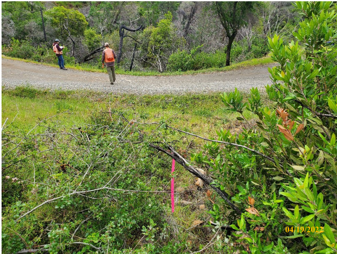
Photo 38. Site 144: View looking downstream towards existing CMP alignment. The CMP is set shallow in the fill and gets filled with sediment reducing its capacity.
