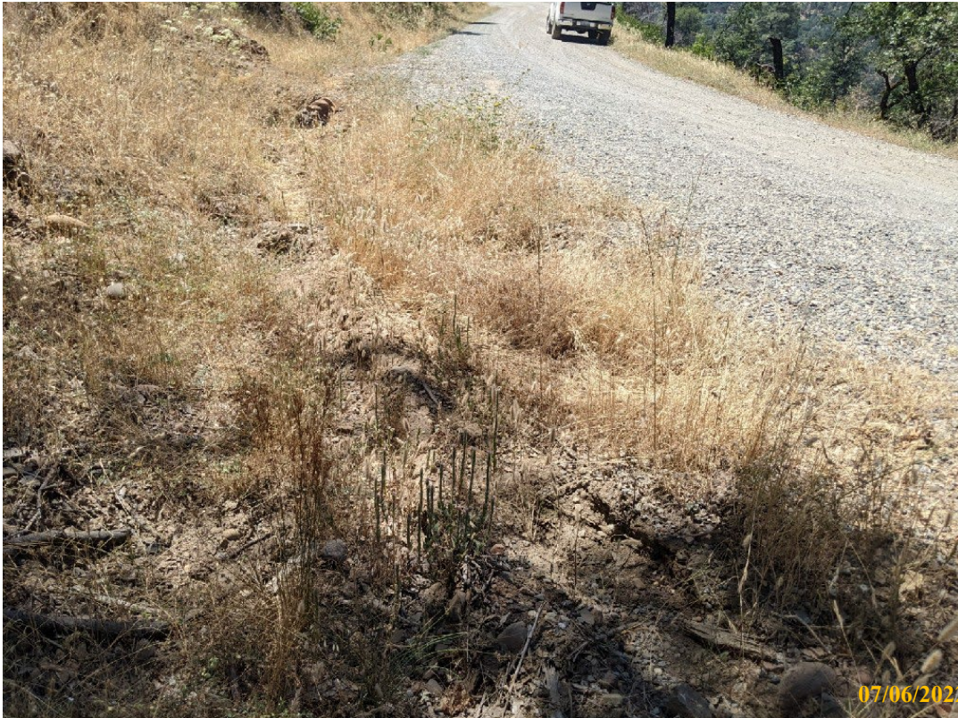
Photo 17. Site 130 : View of inlet of existing DRC#16. The opening of the existing CMP has been crushed.
