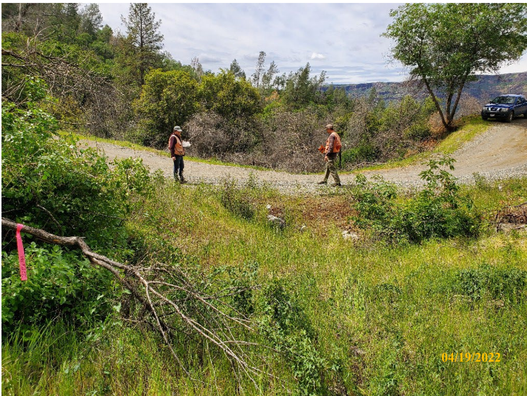
Photo 34. Site 140: View downstream of the current CMP inlet. This CMP transmits long ditch flow and is undersized for this stream.
