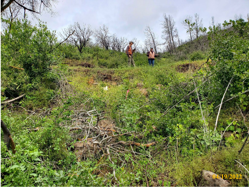
Photo 37. Site 144: View upstream of the outboard fillslope and current shotgun CMP outlet. A new 24-inch CMP will be placed at the base of fill.
