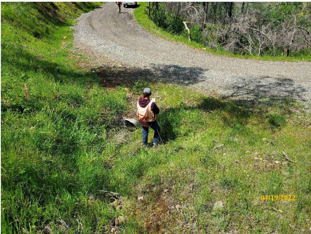
Photo 26. Site 135: View of the current CMP inlet and stream crossing surface from the right streambank. The CMP is partially crushed reducing its carrying capacity and is high in the fillslope on the outlet side.
