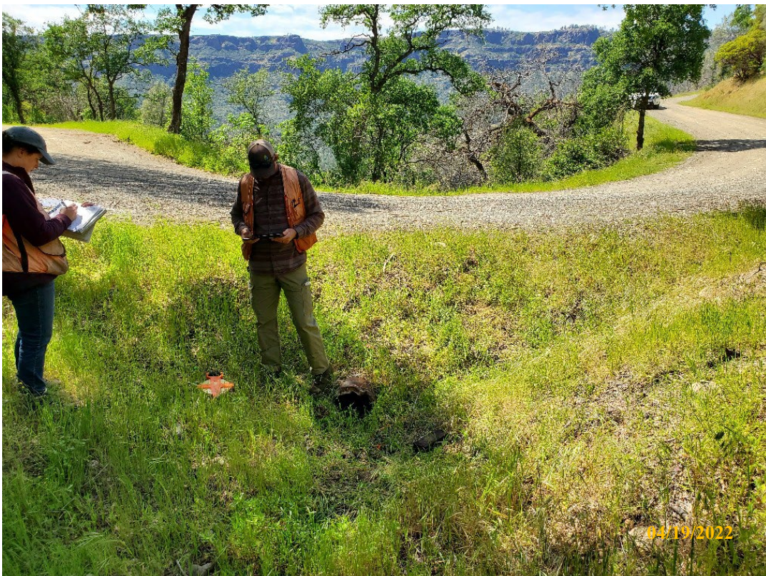
Photo 22. Site 132: View looking downstream at the current CMP inlet and stream crossing surface. The CMP is undersized and delivers long ditch flow from the right.
