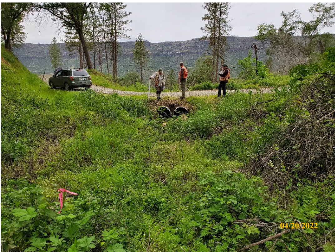
Photo 2. Site 119: View looking downstream towards existing CMP inlets. Both CMPs were recently installed in-kind with the previous undersized CMP. Both CMPs are shallow in the fill and will continue to erode the outboard fill.
