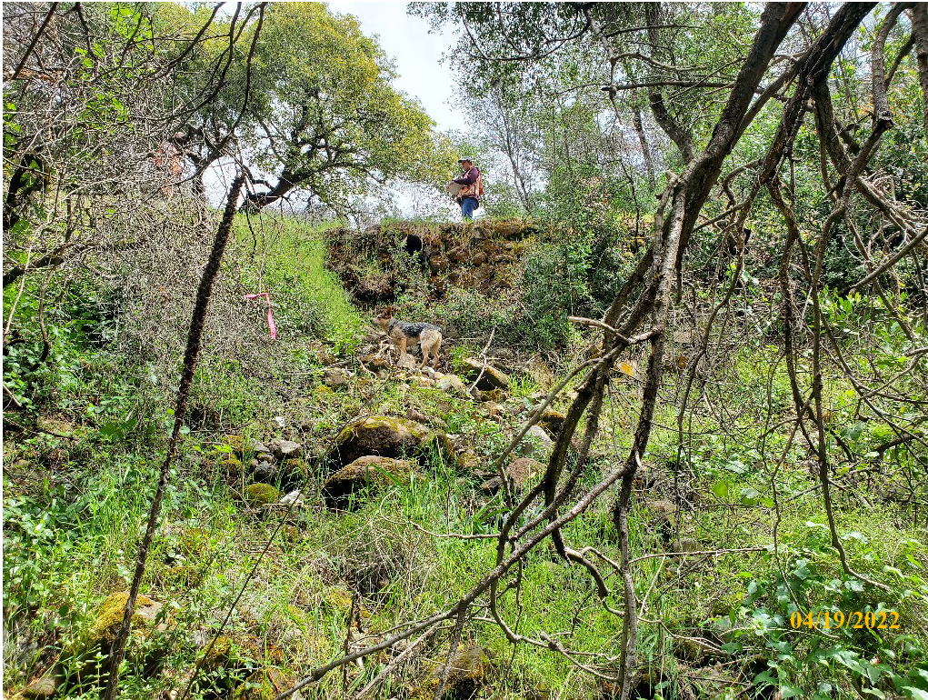
Photo 31. Site 139: View looking upstream at the current CMP outlet and outboard fillslope. A new 30-inch CMP will be placed at the base of fill eliminating the erosion of the outboard fillslope.
