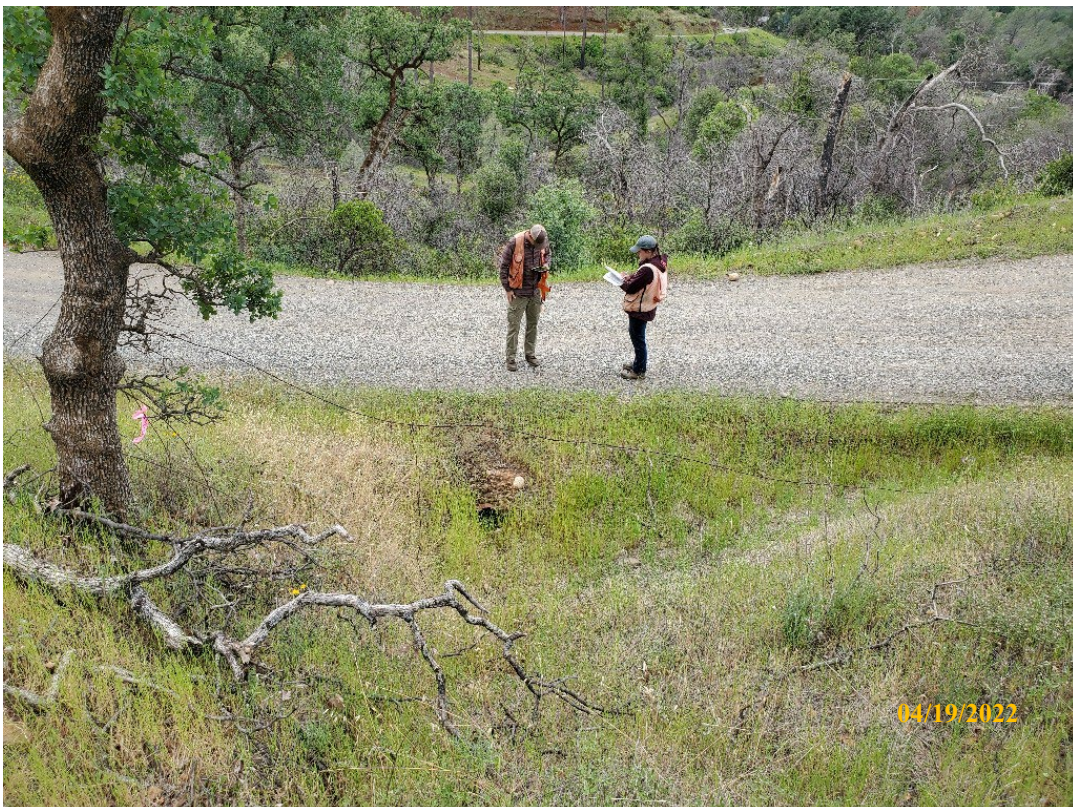
Photo 8. Site 124: View looking downstream at the current CMP inlet and stream crossing surface. The undersized CMP is short and high in the fill and has caused erosion of the outboard fillslope.
