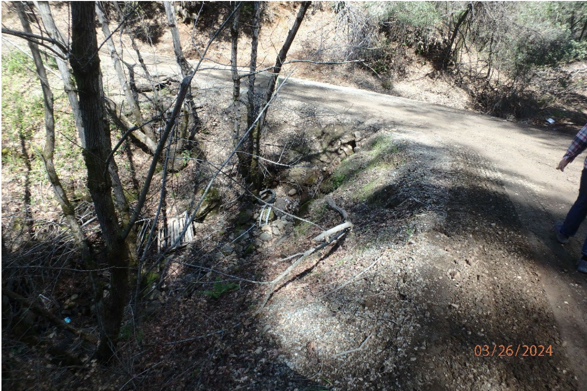
Photo 43. Site 149: View of outboard fill slope and current culvert outlet area. Stream upgrades include installing a new 54-inch CMP at the natural channel grade.
