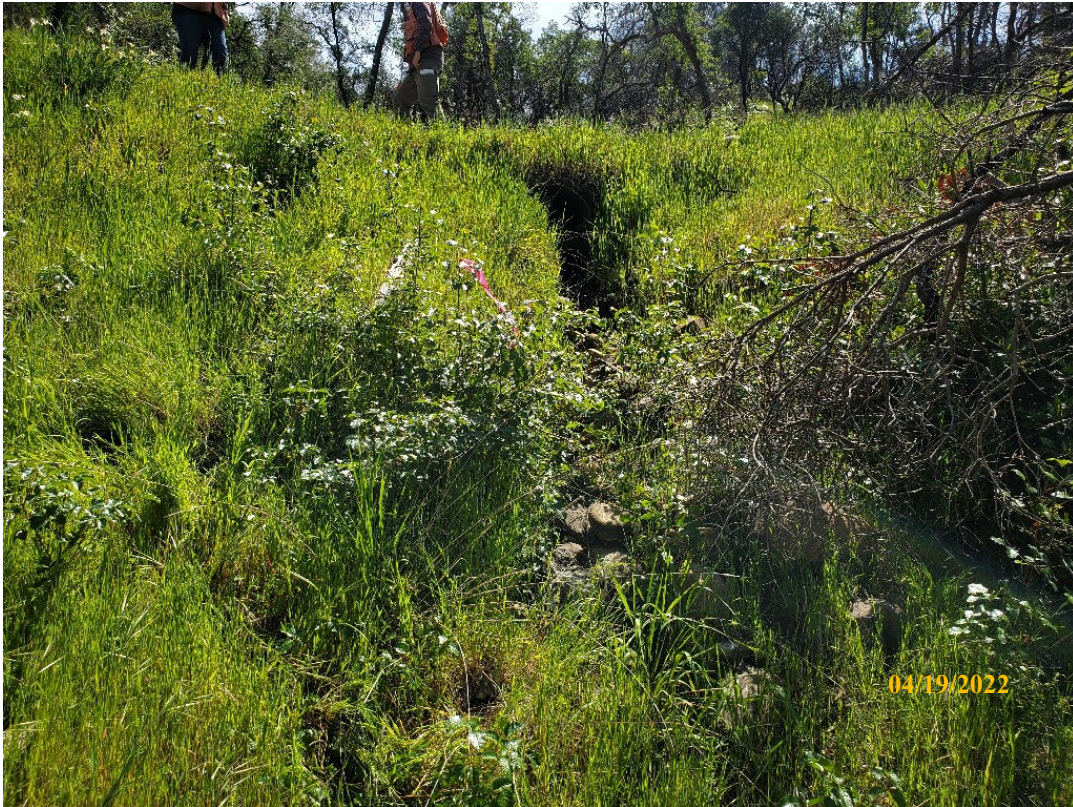
Photo 25. Site 135: View looking upstream at the current CMP outlet and outboard fillslope. A new 24-inch CMP will be placed at the base of fill.
