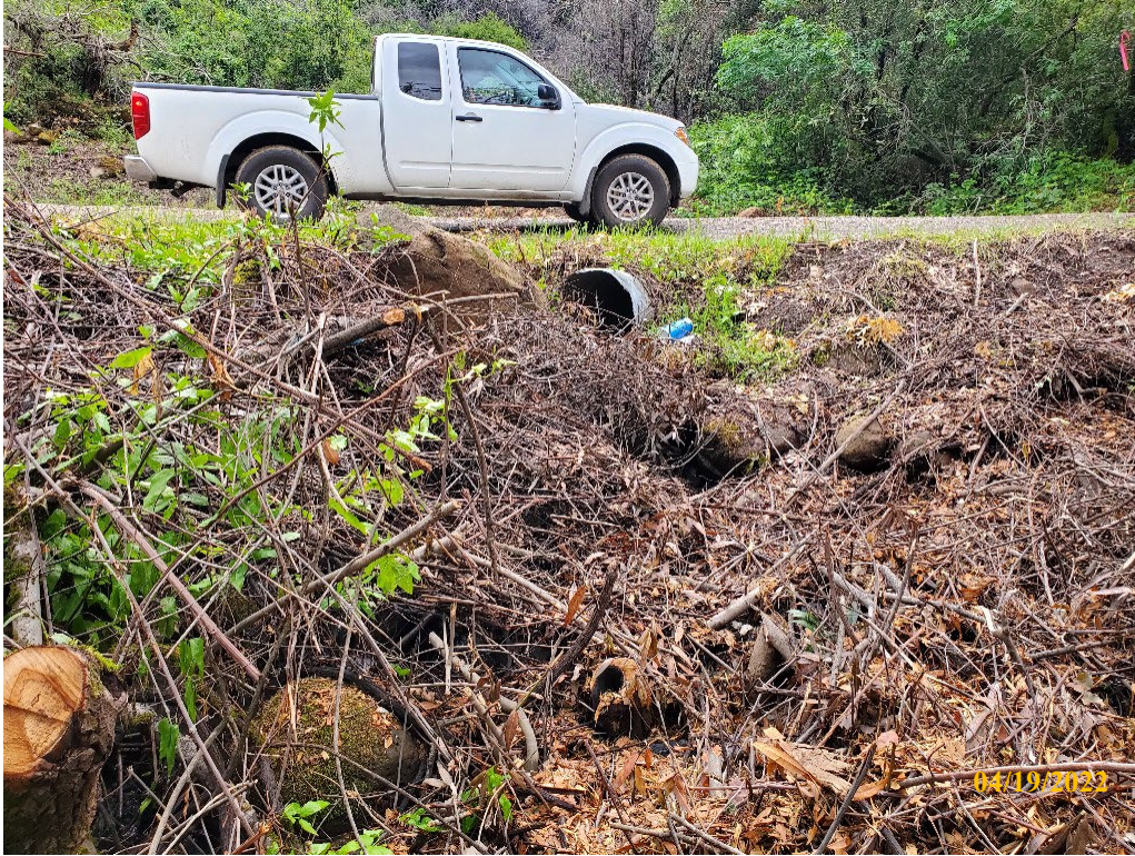
Photo 35. Site 142: View of the current CMP outlet and outboard fillslope. A new 60-inch CMP will be installed at the base of fill and at stream grade to allow for passage of sediments.
