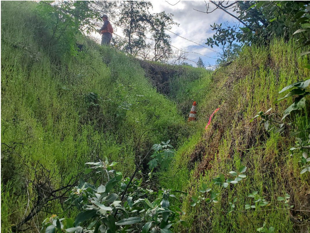
Photo 15. Site 129: View looking upstream at the current CMP outlet and outboard fillslope. A new 24-inch CMP will be placed at the base of fill reducing the amount of future outboard fill erosion.
