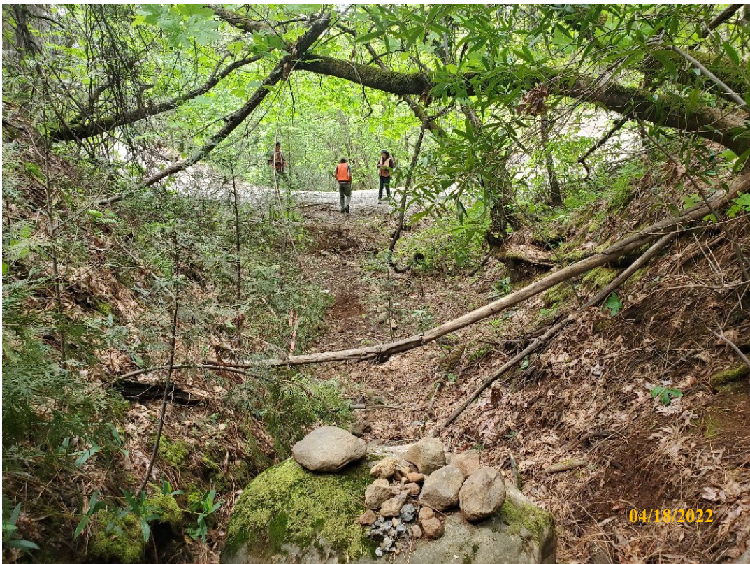
Photo 42. Site 148: View looking downstream towards the stream crossing. The current CMP is undersized and periodically plugs with sediment.
