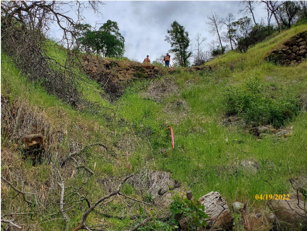
Photo 9. Site 125: View looking upstream at the current CMP outlet and rocked outboard fillslope. A new 30-inch CMP will be placed in line with the channel and set at the base of fill.
