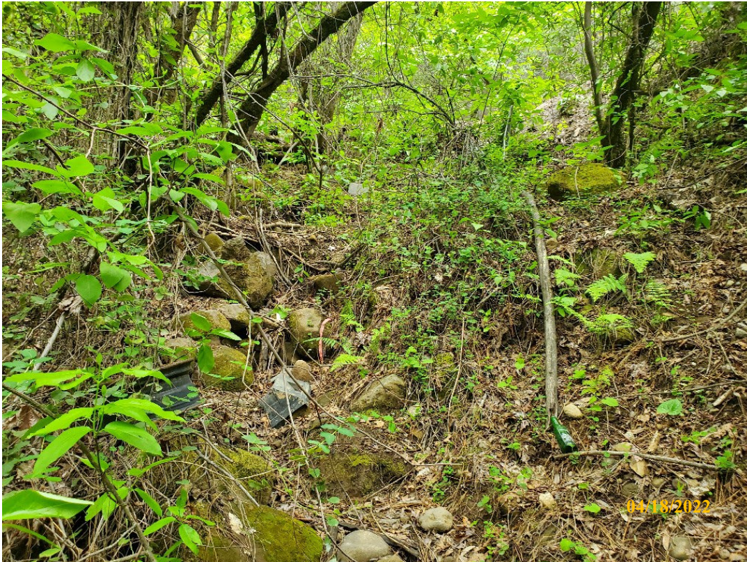
Photo 41. Site 148: View looking upstream towards the outboard fill slope and current CMP alignment. Stream upgrades include installing a new 48-inch CMP and aligning it with the natural channel at grade.
