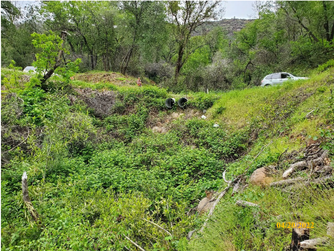
Photo 1. Site 119: View from the left streambank looking towards existing CMP outlet and outboard fillslope. A new 60-inch CMP will replace the double CMPs and will be set at the base of fill.
