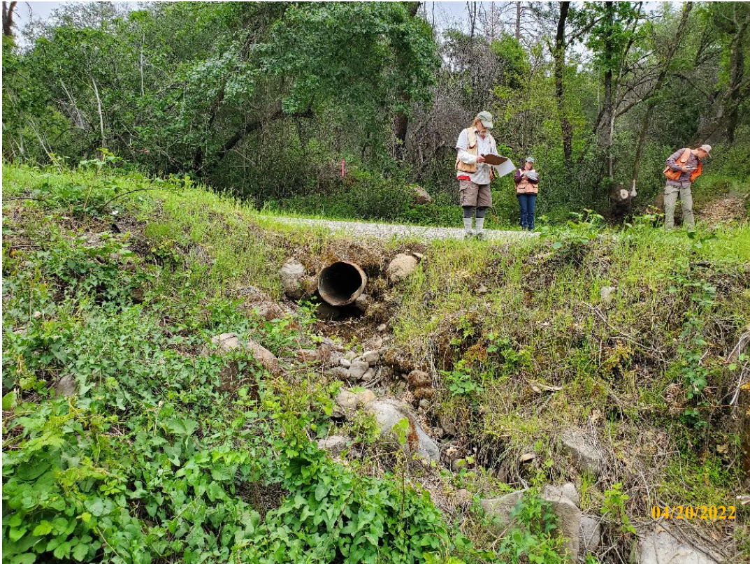
Photo 3. Site 120 : View looking upstream towards existing CMP outlet and outboard fillslope. A new 48-inch CMP will be installed at the base of fill and will be aligned with the stream channel.
