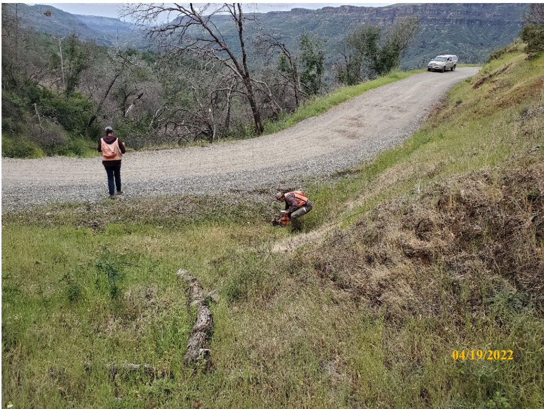
Photo 10. Site 125: View looking downstream. The undersized CMP is not in line with the channel and is set high in the fill. A stone crib wall buttresses the fillslope but is slowly being filled in with sediment from overtopping at the inlet.
