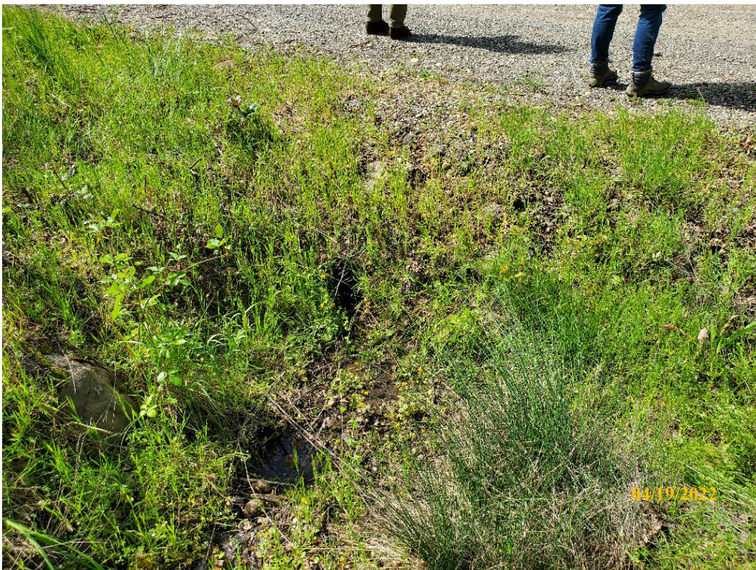
Photo 20. Site 131: View looking downstream at the plugged CMP inlet. The current CMP is undersized and is short in the fill causing erosion of the outboard fillslope.
