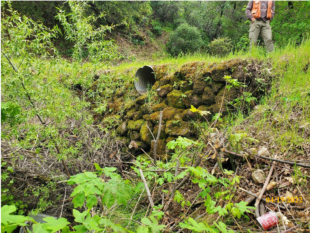
Photo 29. Site 138: View looking upstream at the current channel outlet and armored outboard fill slope. A new 72-inch CMP will be placed at stream grade and aligned with the stream channel.
