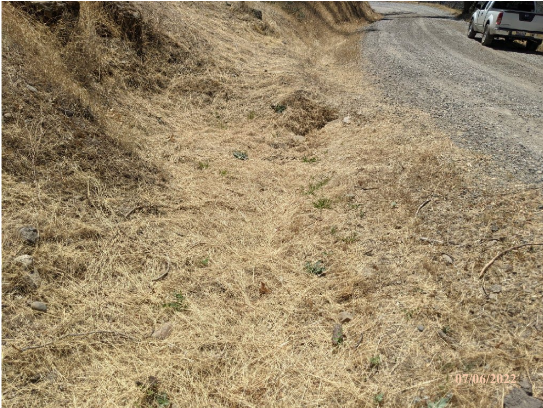
Photo 13. Site 128: View of inlet area of existing DRC#19. Standing in inboard ditch 20 feet uproad of inlet.
