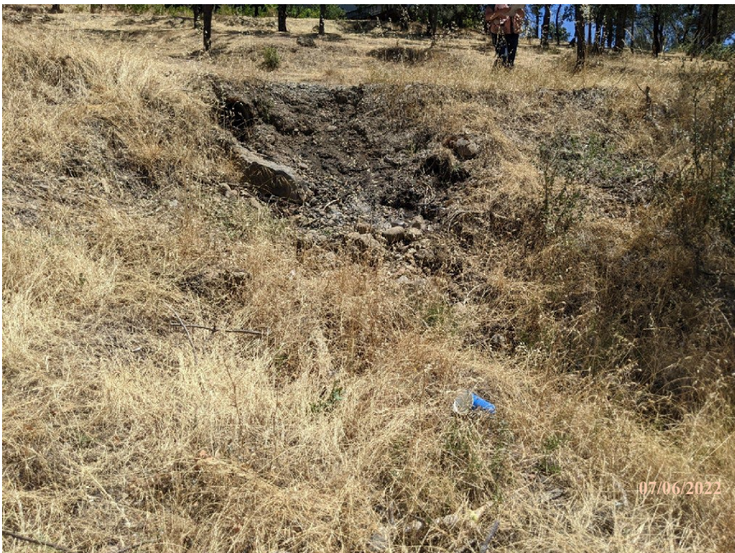
Photo 14. Site 128: View of outlet area of existing DRC#19 from 30 feet below outboard edge of road.
