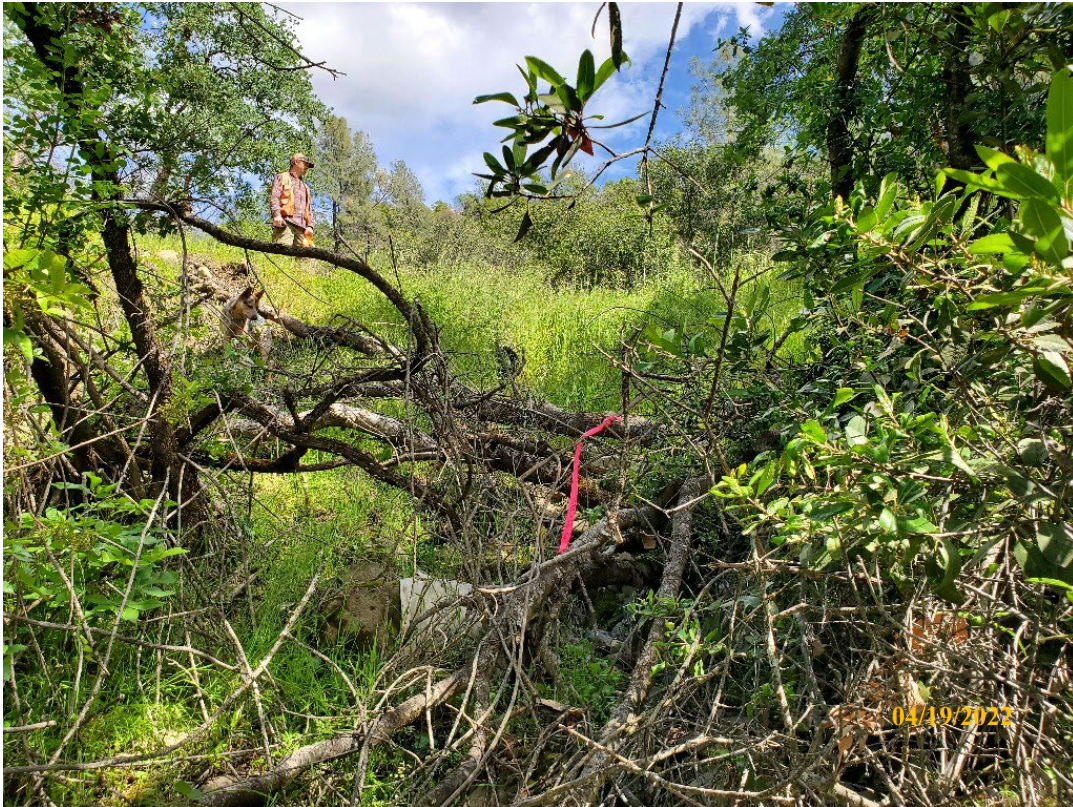
Photo 21. Site 132: View looking upstream towards the outboard fillslope. A new 30-inch CMP will be placed at the base of fill and the long ditch flow will be truncated with the installation of a DRC to the right ditch.
